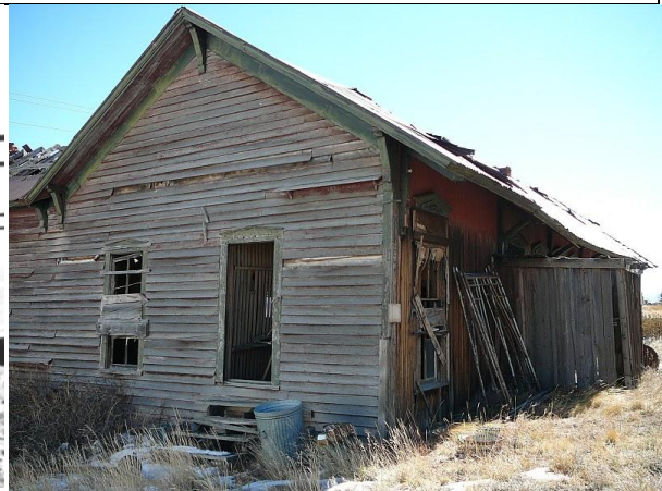
Depot 2008 – most of roof missing, foundations on this side rotted away, in danger of collapse. Later paint scheme still present under eaves. Note original woodwork detail.
