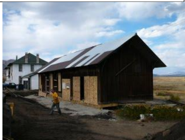
Depot 2009 –structural repairs and new foundations undertaken with assistance of State Historical Fund Grant.
